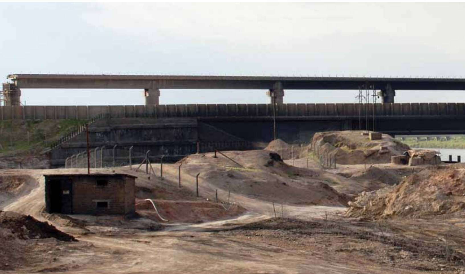
Al Fatah Bridge, with oil pipeline, after insurgent attack, Iraq , 2006. (U.S. Army photo)
