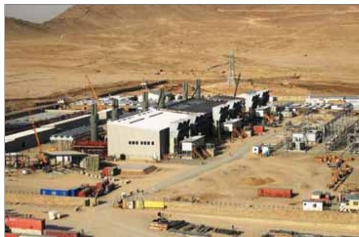
Kabul Power Plant, Afghanistan, 2010. (SIGAR photo)
