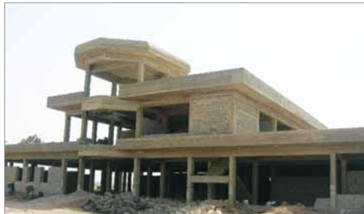
Kahn Bani Sa'ad Correctional Facility, Iraq, at the time of Parsons' termination, 2006. (U.S. Army Corps of Engineers photo)
